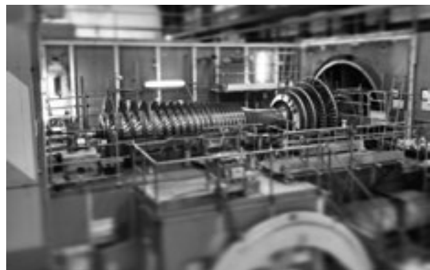
GT13E2 MXL2 first implementation at South Humberbank PS (UK).
